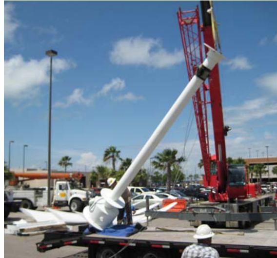
Figure 1: Lifting Axis and Generator
